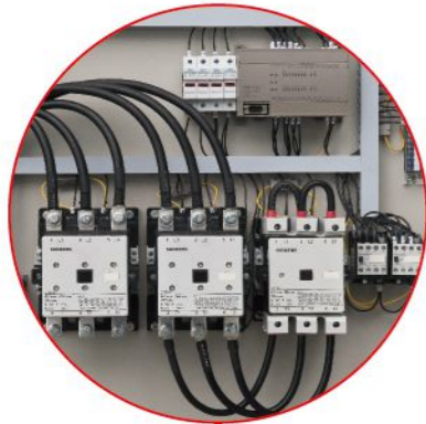
Electricity Board ( Siemens/ABB PLC )
